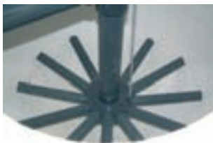
Collector arms detail
